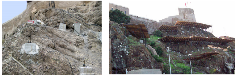
Borehole extensometers and in-place inclinometers installed for online slope monitoring at Al Mirani Fort, Oman
